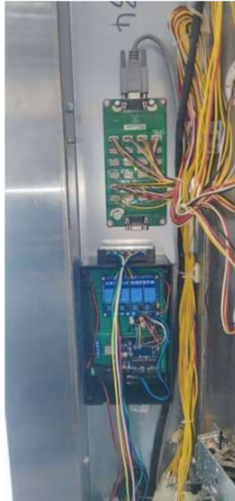
Figure 2. Installed RFID elevator access control module
